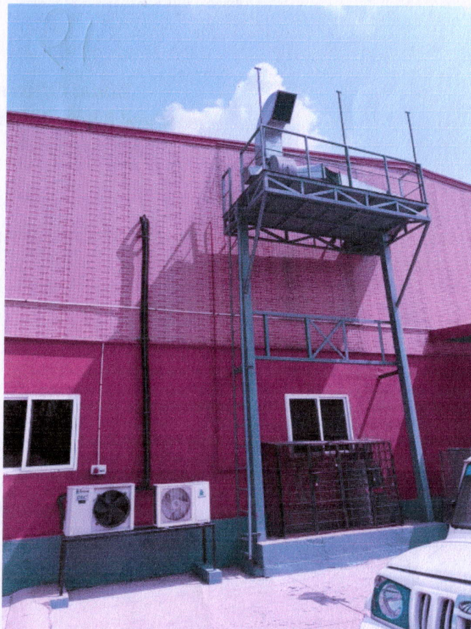
Air handling/ odour control system can be seen installed and operational
